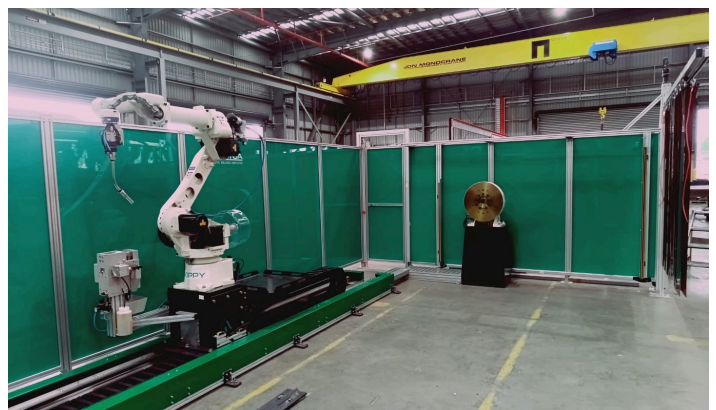
U-6000 robotic welding cell installed in the new facility.
