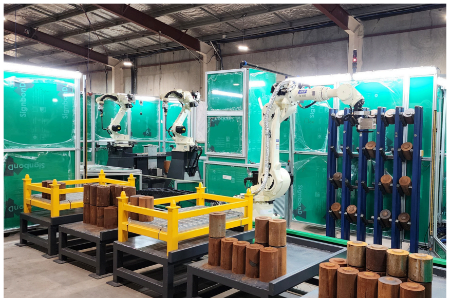
Full View of Anode Yoke Repair Cell with Yoke Loading Stations.
